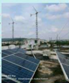
Campus Hybrid Power Plant
